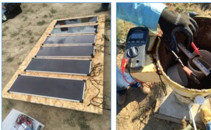
Figure 7. Solar panels as power source for E-Redox ® pilot system and monitoring of electrical parameters
